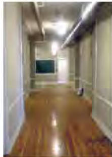
Not Recommended: [66] Interior ductwork has been inappropriately left exposed and unpainted here in this traditionally-finished school entrance hall.
