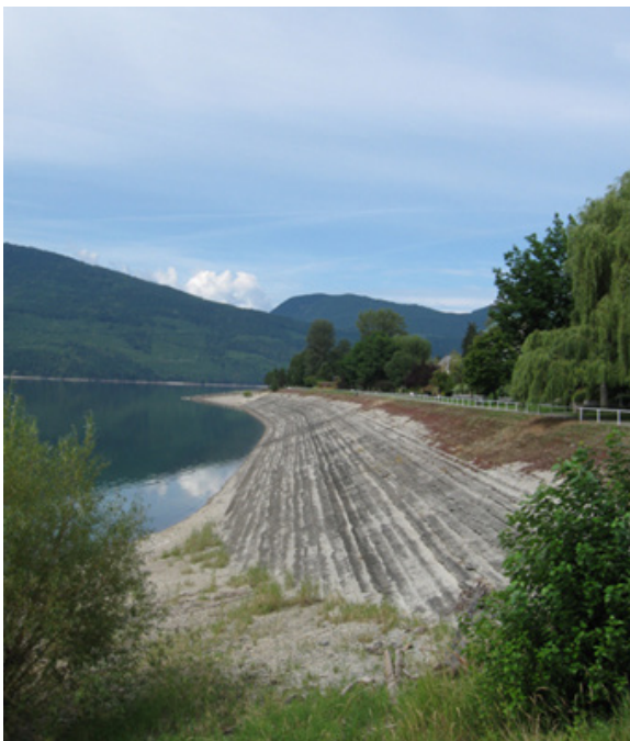
Erosion from a dam reservoir. (Photo: Carolyn Whittaker)
